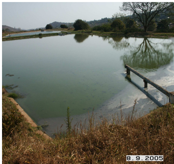
Figure 5: Photo of part of Limbe Wastewater Treatment Plant. The plant uses a pond system.
